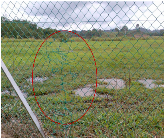
Foto 14 Pagar Dipotong Di Kawasan Empangan Water Treatment Plant
