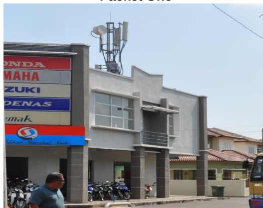
Gambar 4.2 Menara Jenis Roof Top Packet One
