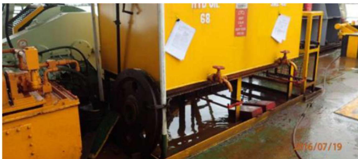
F8.17 Spillage/drip tray provided at fuel/oil container
